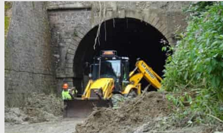
Beaminster Tunnel portal landslide, 2012, 2 dead
